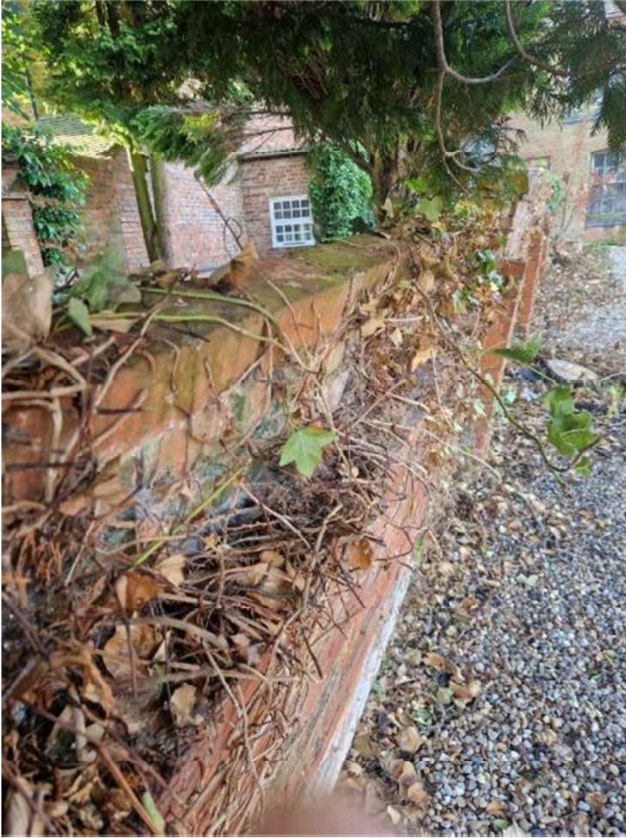
Trees are having a severe impact on the wall.
