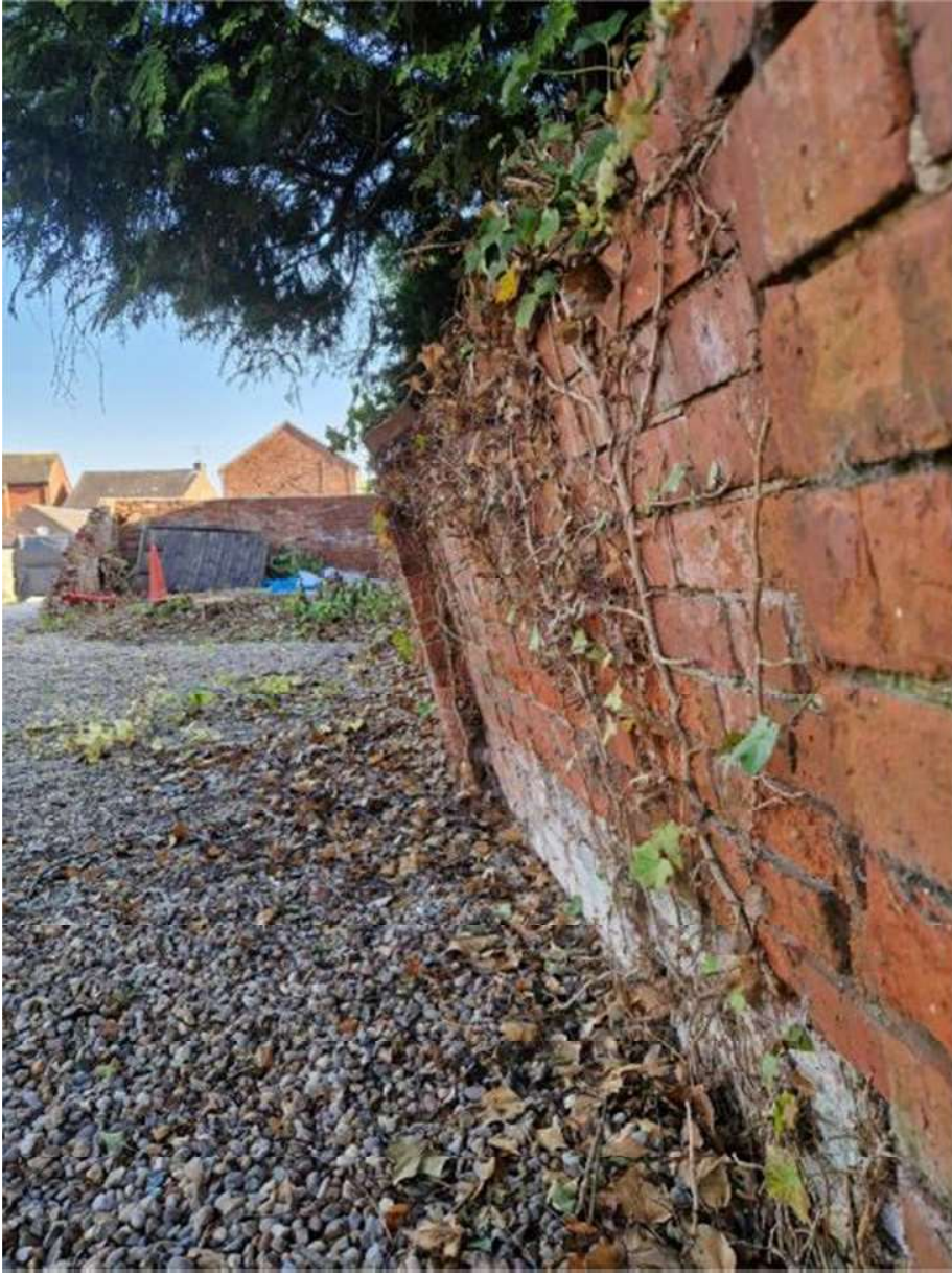
The wall is leaning at such an angle that it is unstable.
