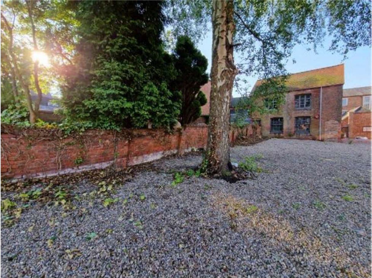
Tree outside the wall line are also influencing the wall stability.
