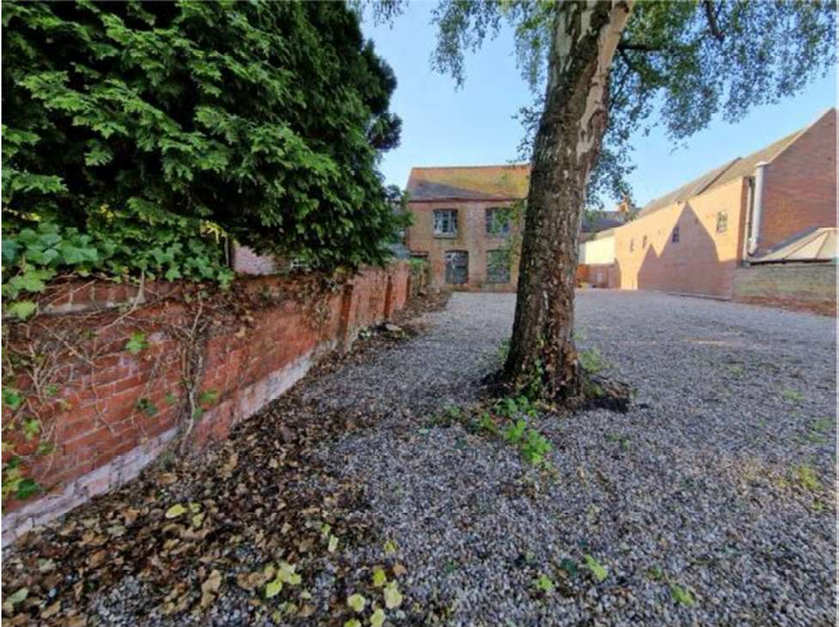
Tree is very close to the wall causing it to become unstable.
