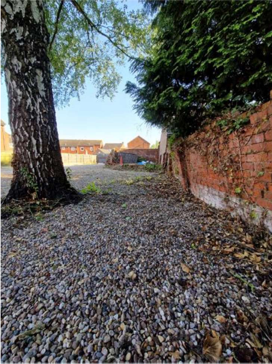
The wall is in a distressed state.
